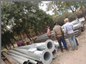
12.5 Meter High Mast Pole LED Street Light
