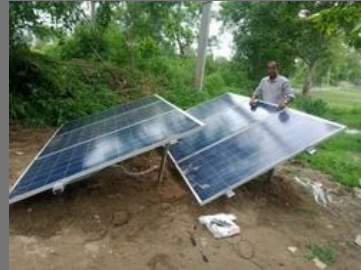
Off Grid Solar Power Plant
