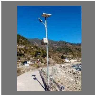
Solar Street Light
