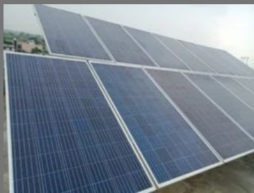
On Grid Solar Power Plant
