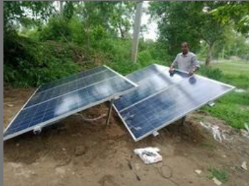
Solar Power Plant
