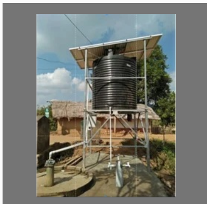
Solar Water Pumping System
